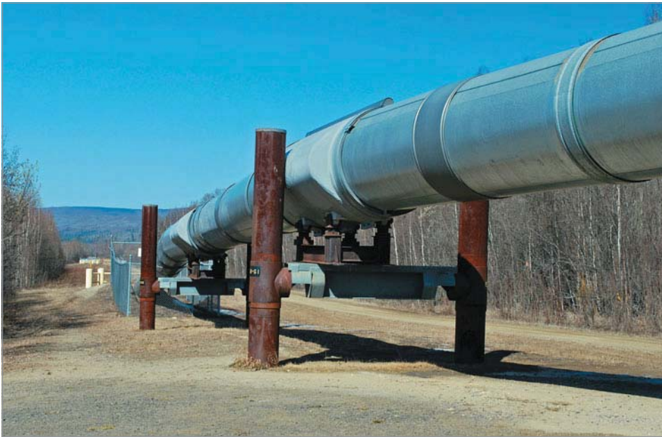
The Trans Alaska Pipeline System traverses 800 miles from the North Slope of Alaska to the northern most ice-free port of Valdez, Alaska. The pipeline is 48 inches in diameter, has 11 pump stations, and has a maximum throughput of 2 million barrels per day.
